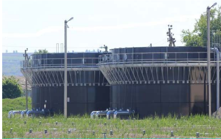
Figure 3. Zone of water filtration through the reed, and water storage tanks [3].
